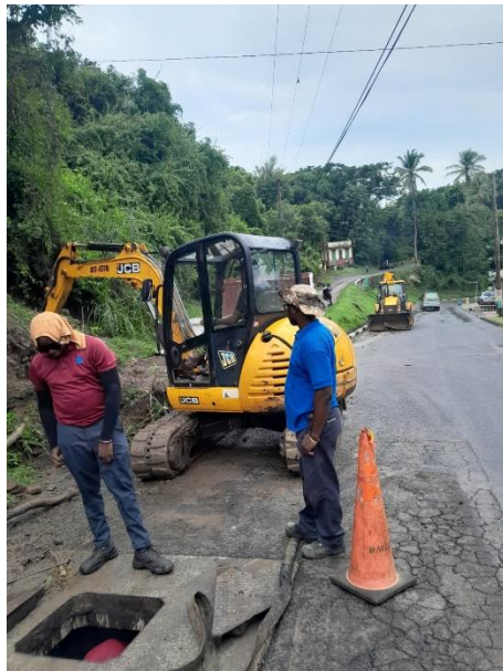
Figure 6. Damaged pipeline in St. David
