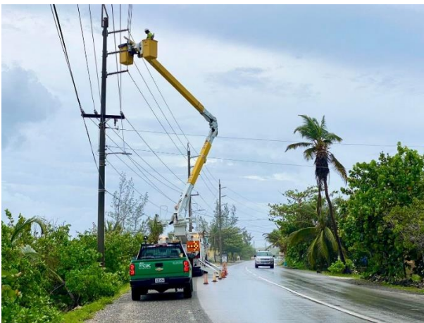
Figure 5 Utility crews supervise electricity lines near Frank Sound. – Photo: Dana Kampa
